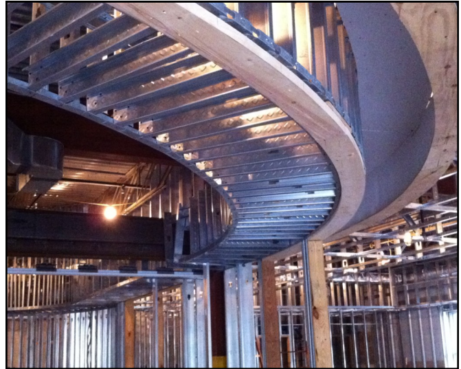
Aries Systems, Inc. new office suite build out, 2012 N. Andover, MA Architectural Design Concepts, Inc., Architect
